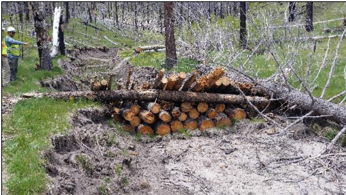
Figure 8. Erosion Control Structures in New Mexico.
