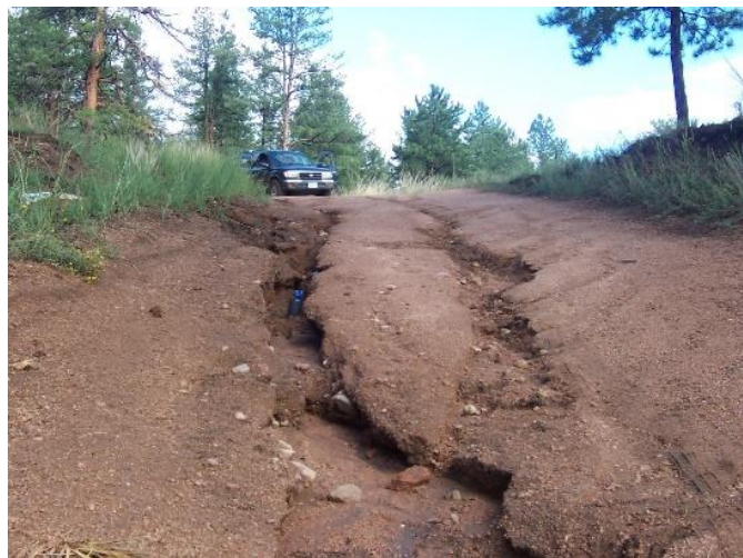
Figure 2. Rills formed on an unpaved road segment in the Sierra Nevada of California due in large part to the steeper slope of the segment and the lack of proper drainage design. This road segment would require relatively frequent grading to remain drivable by normal vehicles at reasonable speeds.
