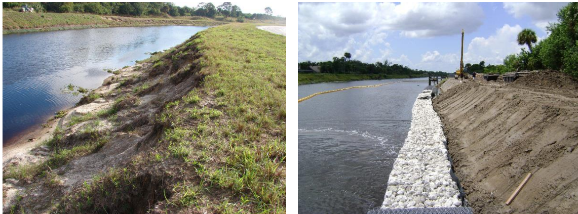
Figure 5. C-24 Canal bank erosion issues and repairs
