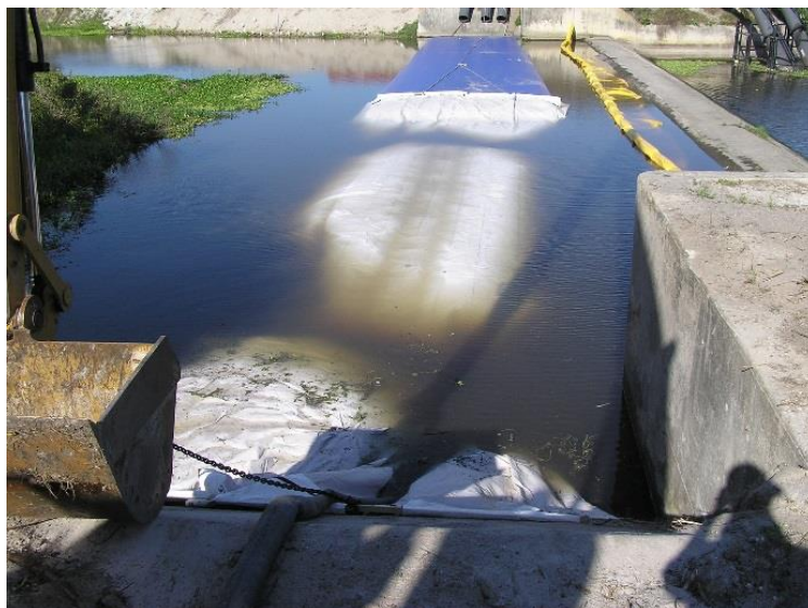
Figure 7. Sediment accumulation upstream of the lateral inflow weir shown in Figure 6
