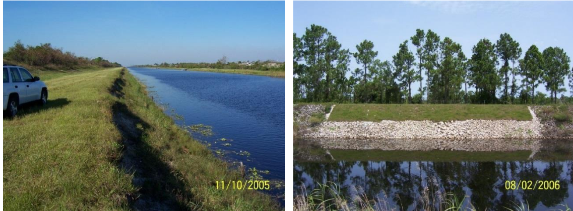
Figure 4. C-23 Canal bank erosion issues and repairs
