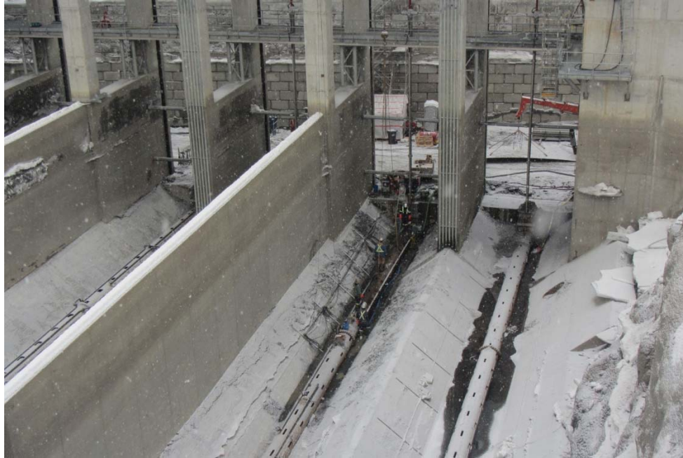
Figure 3. Air purge system being installed along desander sediment collection pipes. Each slot in the larger pipe is equipped with an air nozzle that blasts material off the sediment collector pipe.
