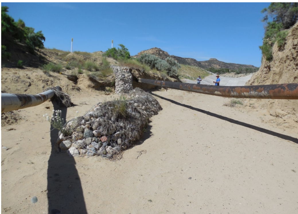
Figure 1. Exposed gas lines as a result of channel degradation in New Mexico
