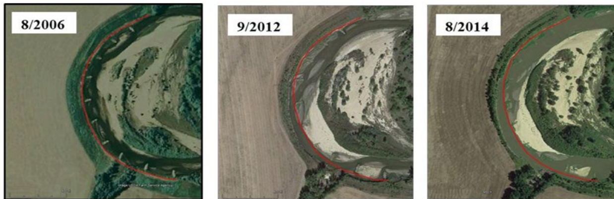
Figure 2. Flanking of rock vanes on the Republican River, KS failed multiple structures within 6 years and all the structures within 8 years. Flow is from top to bottom. From Williams and Shelley (2020).
