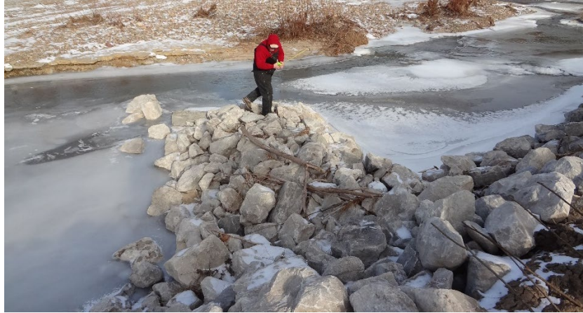
Figure 5. Rock was too small in this bendway weir near Missouri HWY 617. Rock is washing away from a single, moderate flow event. January 2012.
