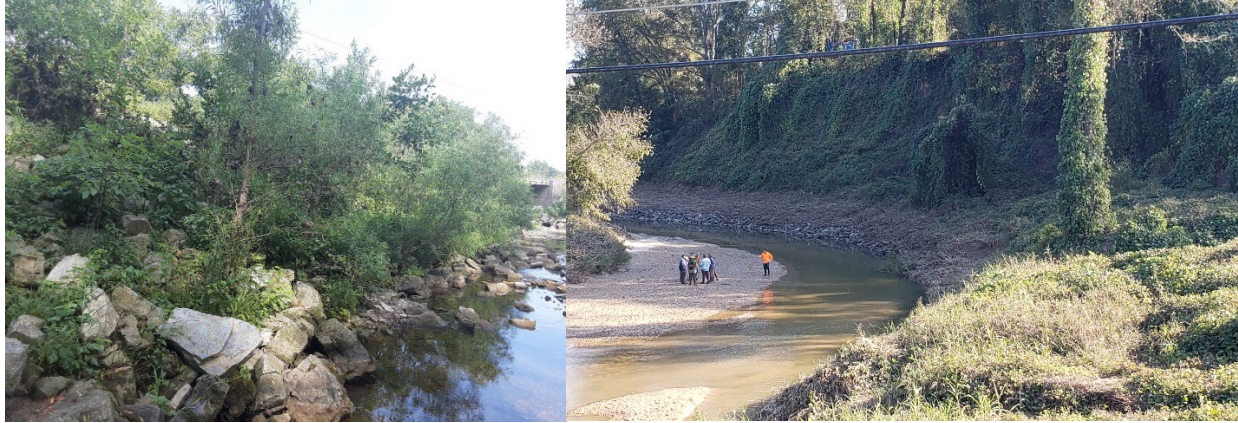
Figure 1. (Left) A whole bank riprap revetment in process of vegetative colonization. Wolf Creek, Missouri. (Right) A whole bank riprap revetment colonized by invasive kudzo. Clear Creek, Mississippi.
