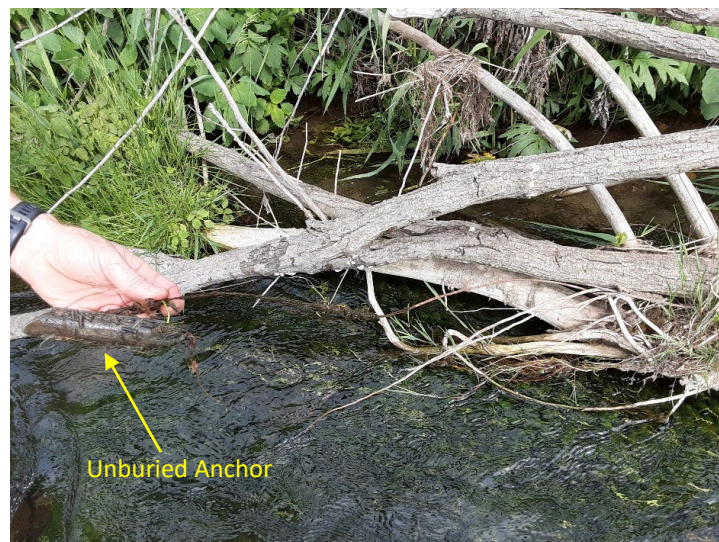
Figure 6. Flanking of a cedar tree revetment on Riceford Creek, MN has eroded so far that the anchor is no longer buried and water flows behind the tree.
