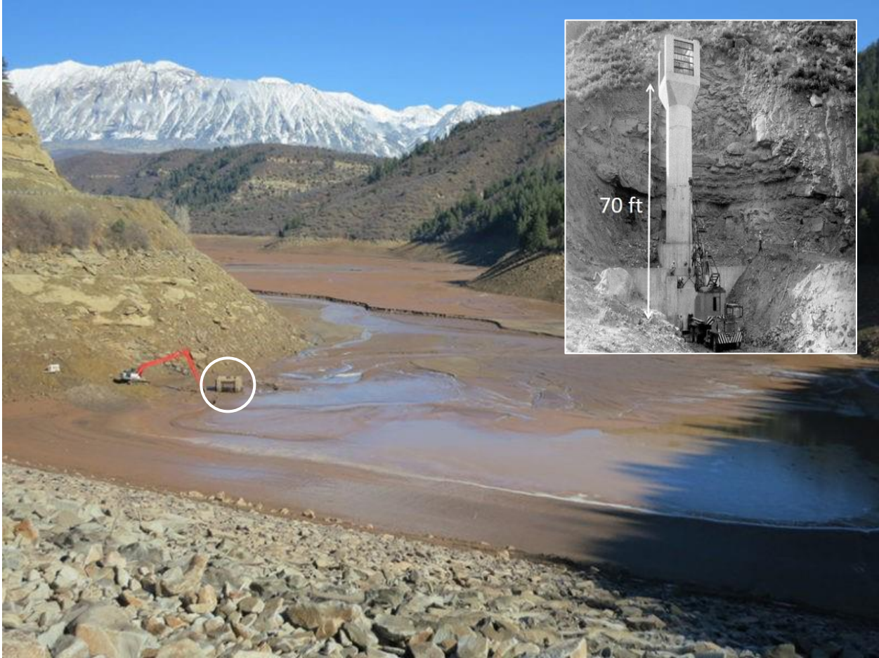
Figure 1. Paonia Reservoir in northwestern Colorado with circled top of outlet structure (2014, large picture) and outlet structure (1961, small picture); source: U.S. Bureau of Reclamation
