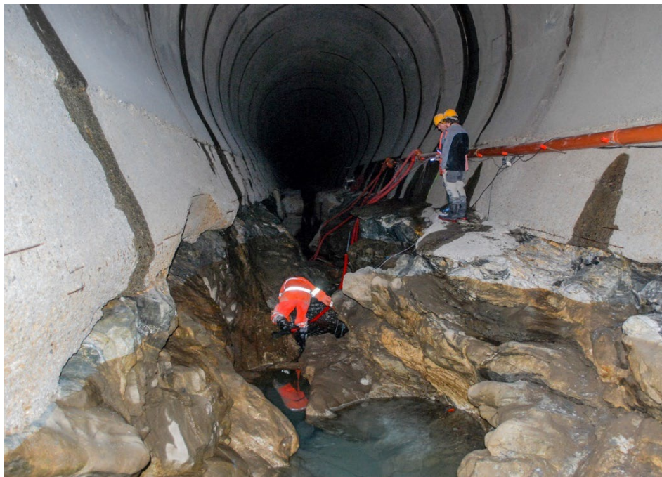
Figure 3. Invert damage in Palagnedra SBT, Switzerland. Horseshoe tunnel cross section with deep abrasion channel (courtesy C. Auel).
