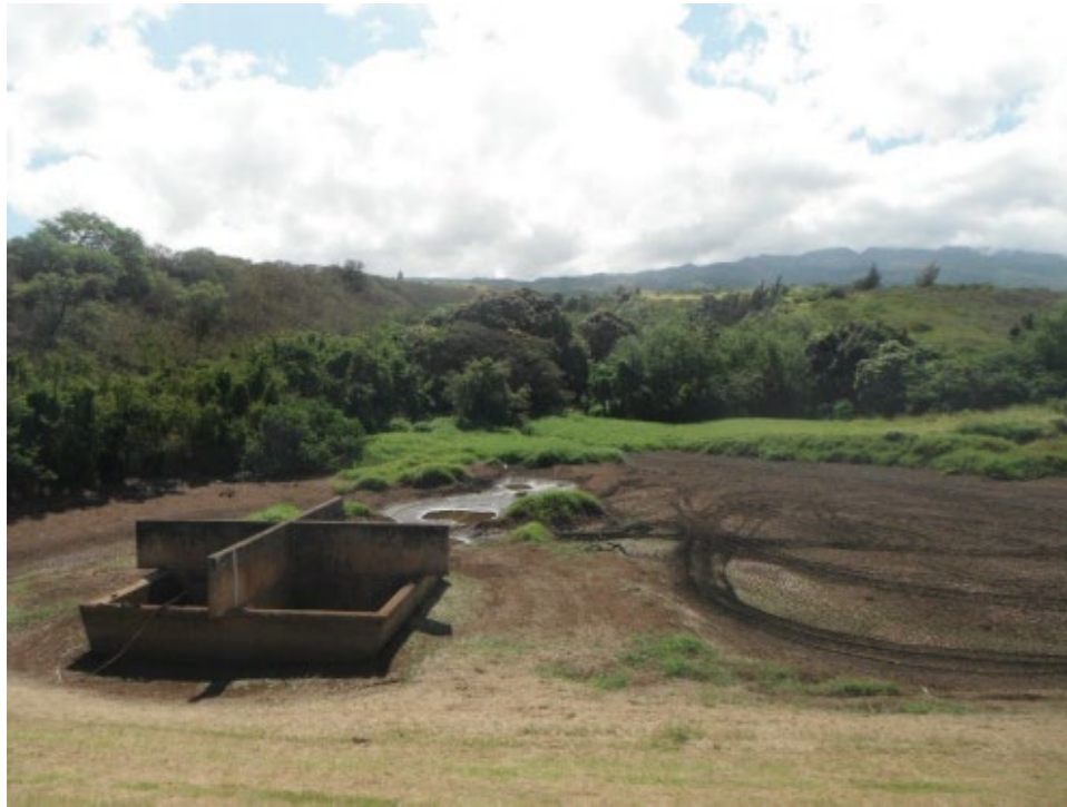
Figure 10. Riser structure and saturated conditions, Kahana Dam
