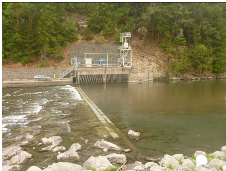
Figure 2. Photograph of the concrete weir and impact plate system mounted to the downstream side. The intake structure is in the background. Flow (approximately 11.3 \text{ m}^3/\text{s} ) is from right to left in the photograph (Sep. 2017).
