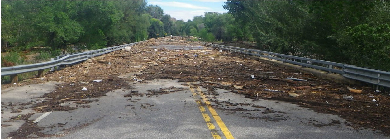
Figure 1: US-34 over the Big Thompson River, CO, just after a 100-year (and expected flood potential) discharge event peaked in an area with increasing trends in both the magnitude and frequency of large floods (9/13/2013).
