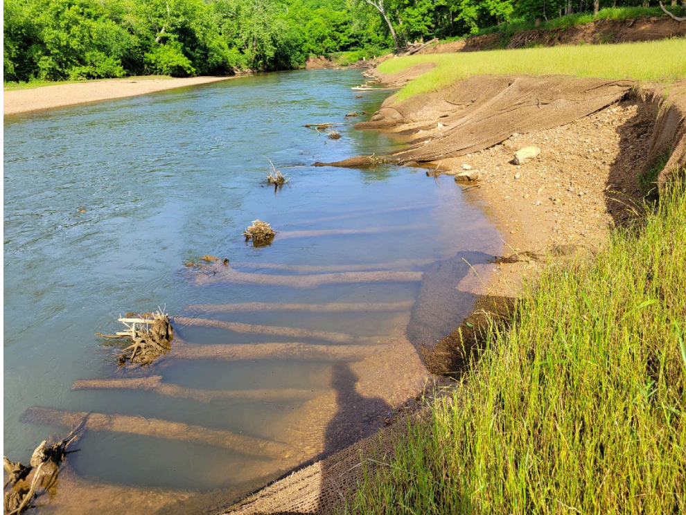
Figure 27. Bank 3 monitoring – scour above one section of toe wood. Facing downstream.
